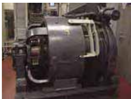
Figure 1 A lift motor
