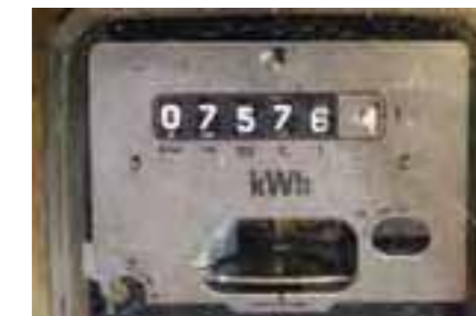
Figure 2 An electricity meter
